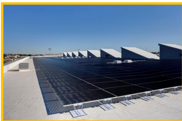
Figure 1-13 Panneaux photovoltaïques. www.ArchDaily.com
