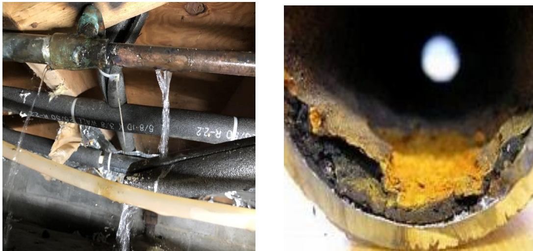
Figure I.2: examples of H_2S corrosion on pipes [16].
