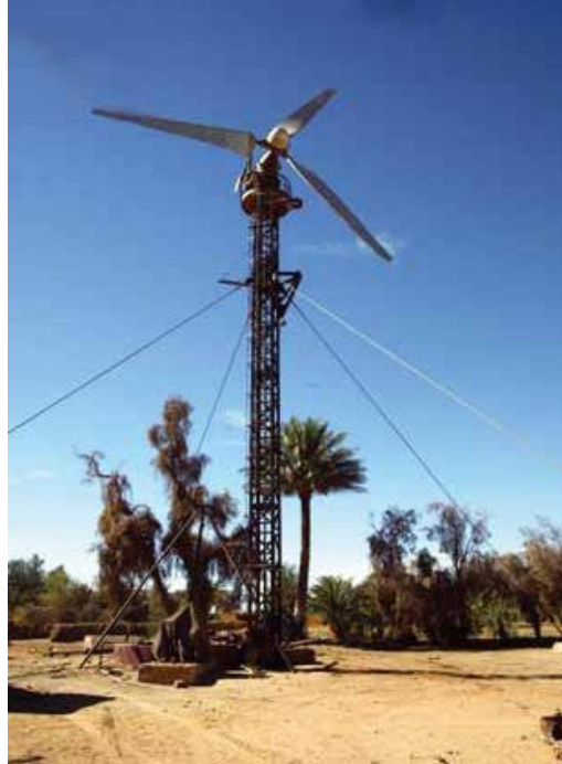
Fig. 23: Wind pump in Adrar
