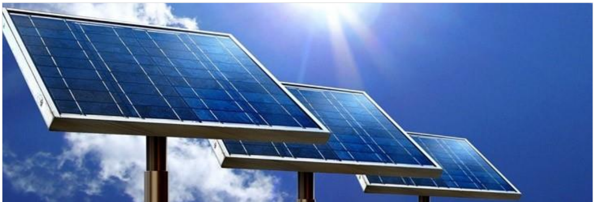
Figure 133 : Panneaux photovoltaïques, www.google-image.com
