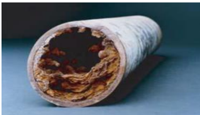
Figure.I.23: Pipeline affected by MIC corrosion
