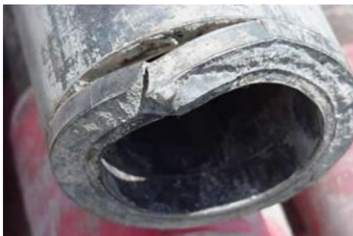
Figure.I.22. Oil and gas pipeline under sour corrosion
