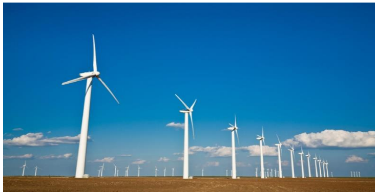
Figure I.3 : Horizontal-axis wind turbines on a wind farm [7].
