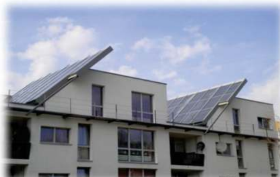
Photo 17: les panneaux photovoltaïques Source : http://www.pizzatravel.com.ua/eng/germany/9/kronsberg_district_in_hannover
