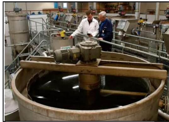
Figure I. 31 station de traitement des eaux usées. Source: http://web.worldbank.org/archive/website01419/WEB/IMAGES/CITY_S-2.PDF
