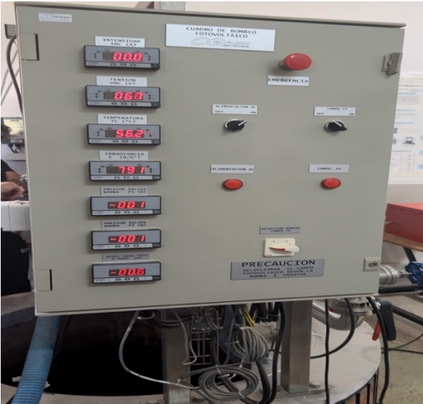
Figure III. 4 : Power Conditioning Unit (PCU) in URAER.
