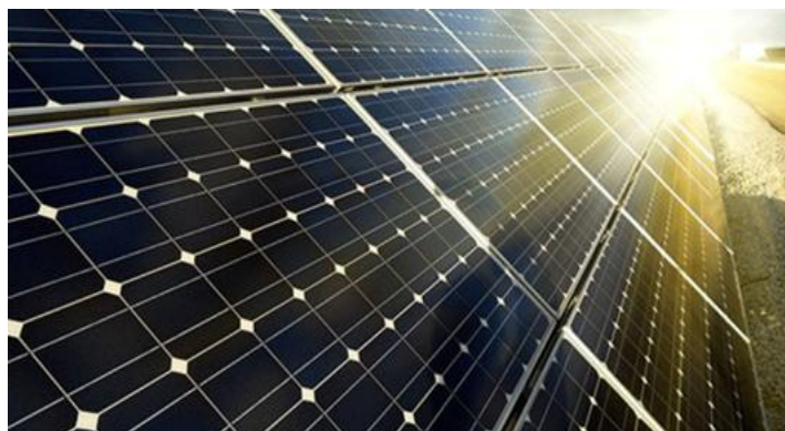
Figure I.3: panneaux solaire photovoltaïque [1]
