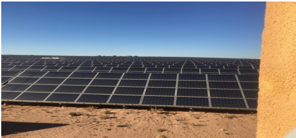
Figure 2.3: Polycrystalline Silicon Solar Panel of SKTM, Laghouat, Algeria.
