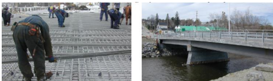
Figure 2.32 : Tablier de pont en PRFV, Cookshire-Eaton – Quebec
