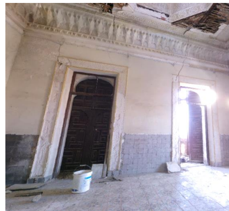
Figure 75 : fissures , source : scanner BLK360 Sahli
