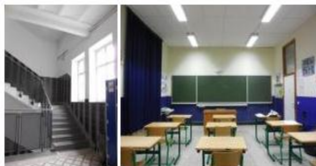
Figure V-12: Murs soumis aux salissures.
