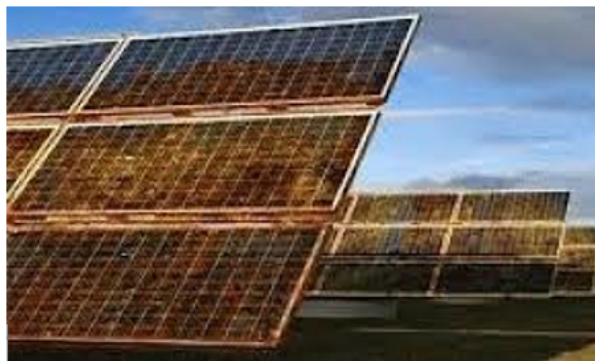
Figure 2.4: corrosion in solar cell (35)
