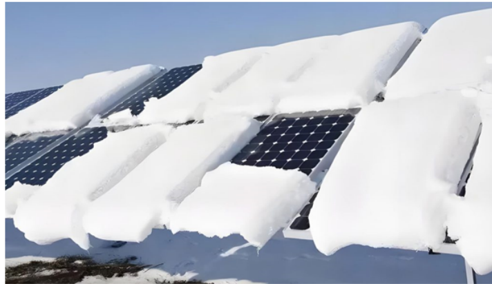
Figure 2.13: Solar PV panel full covered and partially covered by snow
