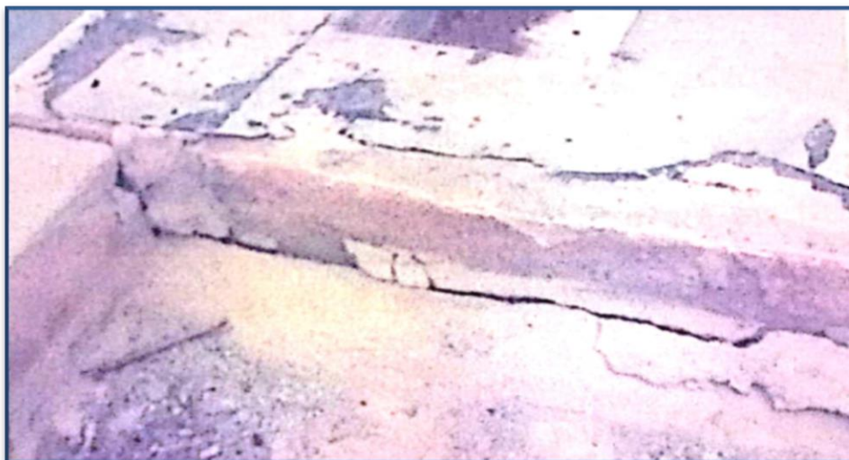
Figure II.33 : Joint mal traité plancher terrasse [44]
