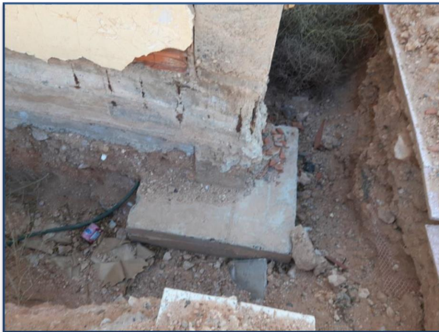
Figure II.32 : Corrosion des armatures transversales. [44]
