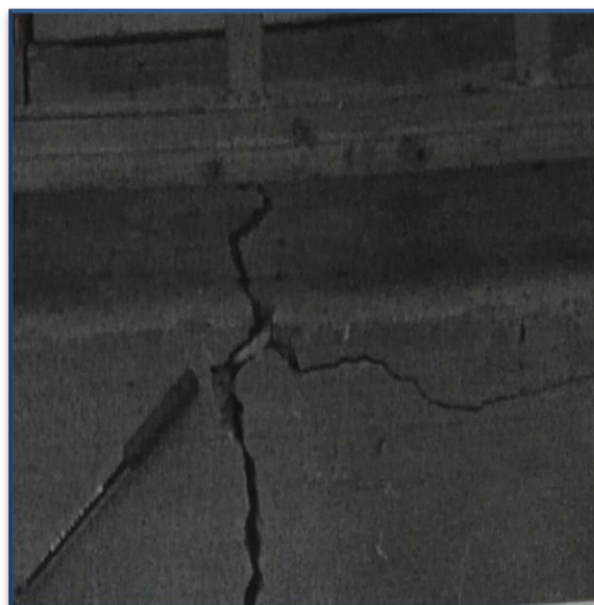
Figure II.28 : Eclatement et fissuration [44]
