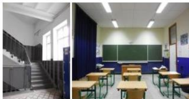
Figure V-12: Murs soumis aux salissures.
