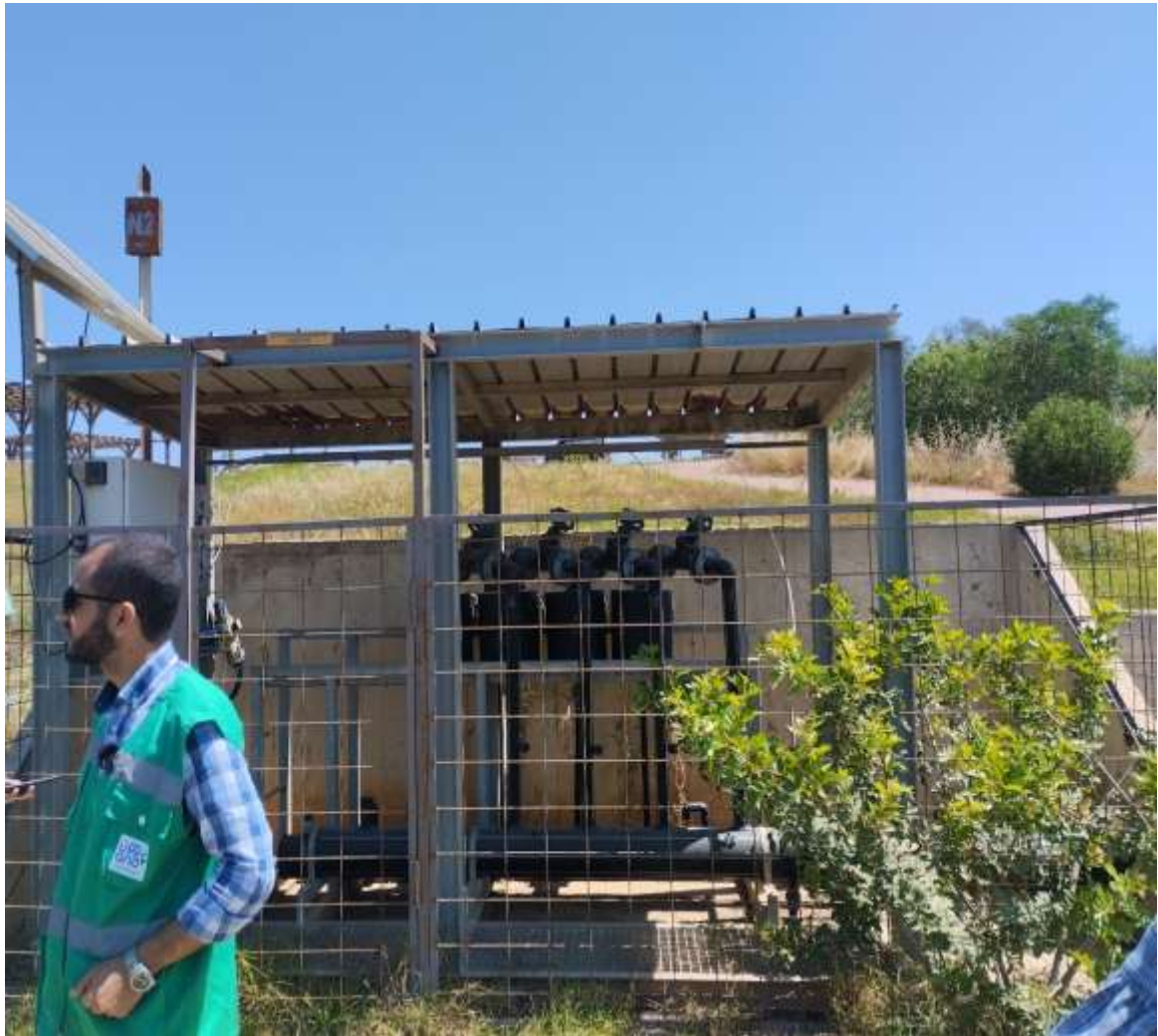
Figure 33 Electricity Cogenerator (Benaissa, 2023)
