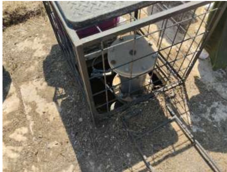
Figure 32 Biogas and leachate pumping well (Benaissa, 2023)
