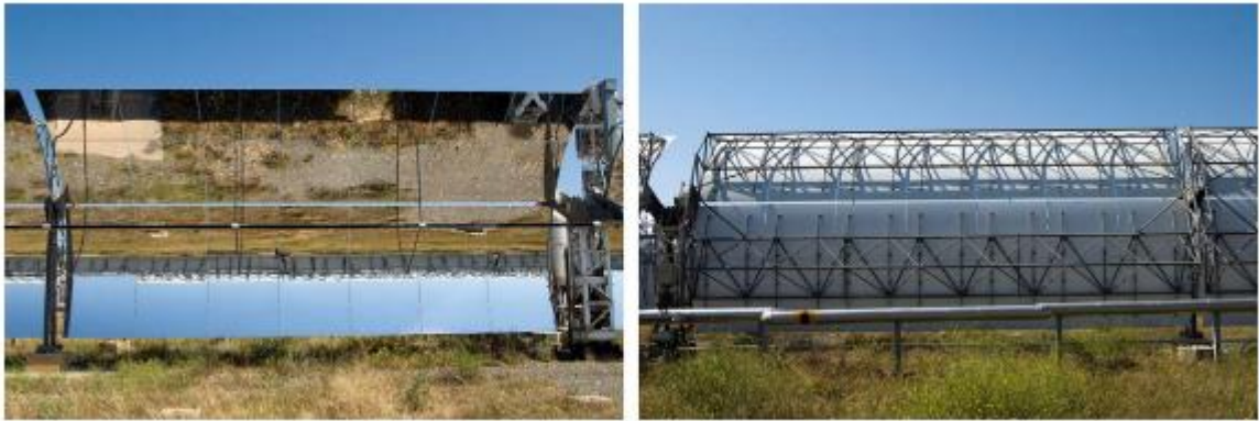
Figure I. 14. Front (left) and rear (right) views of LS-3 collector.
