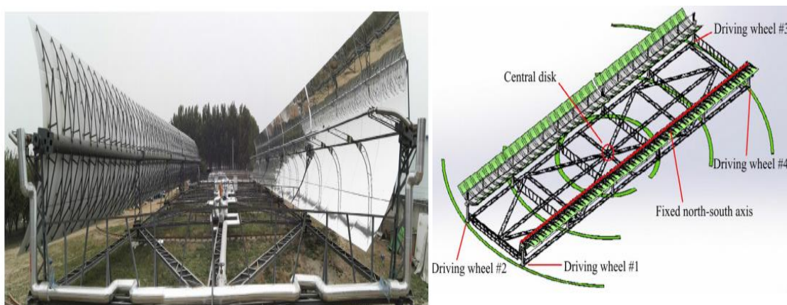
Figure I. 24. Photo of the 300-kW solar parabolic trough collector with rotatable axis tracking Schematic of the rotatable axis tracking apparatus [51]
