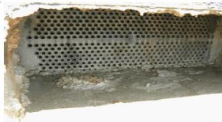
Figure II .4): deposit of bacterial slime, hydrocarbons and metal oxides in a heat exchanger water hydrocarbon (petroleum refinery).
