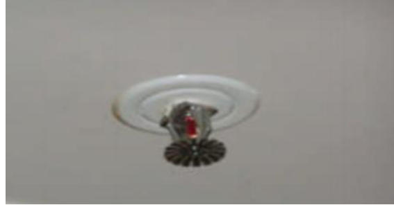
Figure 139: SPRINKLERS. Source: http://ww2.ac-poitiers.fr
