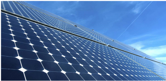
(a) solar panels.[18]
