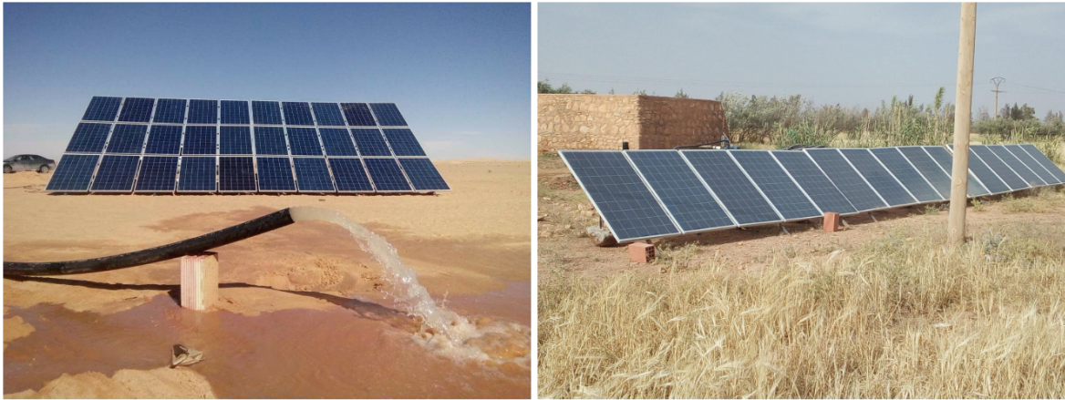
Solar irrigation by Mekk Energy, Sidi Makhlouf region, Laghouat.
