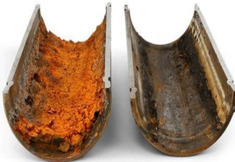
Fig II.3 : internal corrosion defect
