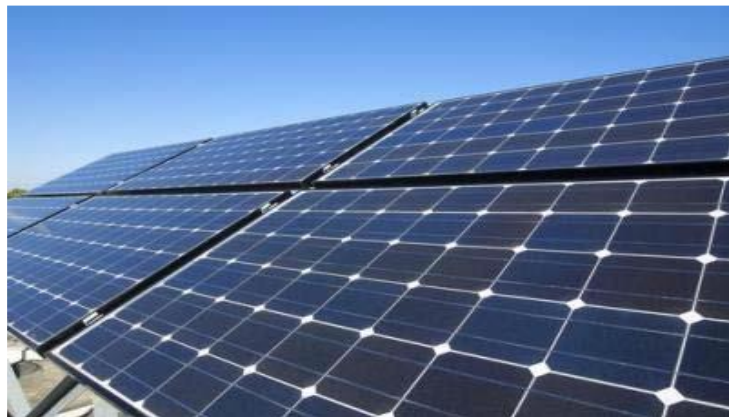
Figure I- 1: example of PV field.
