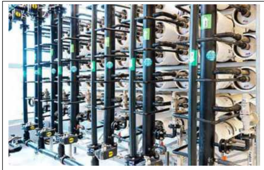
Figure (2.12): Prototype de centrale osmotique (Statkraft) Ref: [20]
