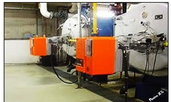
Figure 19: chaufferie centrale. Source : www.energieplus
