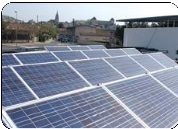
Figure n 24Les panneaux photovoltaïques /source: projet urbain-AZZAG
