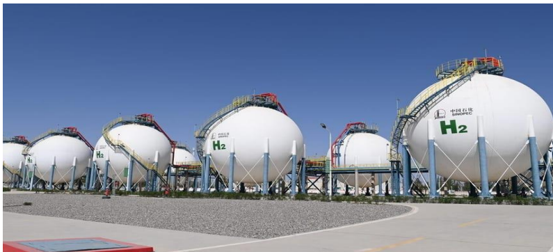
Figure 1.3: Liquid Hydrogen Tanks
