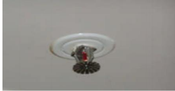
Figure 139: SPRINKLERS. Source: http://ww2.ac-poitiers.fr
