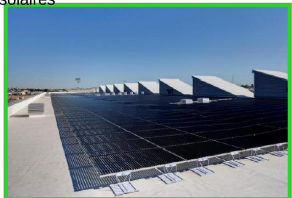
Figure 22:Panneaux photovoltaïques. Source : www.ArchDaily.com
